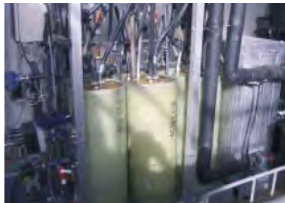
Fig. 2: Five desalination modules are in operation in the two-loop system on Gran Canaria. The collector field has an area of 90 m 2 and consists of flat-plate collectors equipped with a double-glazed cover with anti-reflective coatings. This allows a good efficiency value of 50 – 60 % to be achieved even for high operating temperatures of 80 – 100 °C. The thermal storage tank has a volume of 4 m 3 .
